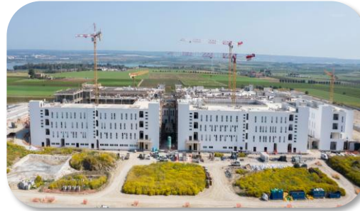
2017-2025 New Hospital San Cataldo di Taranto Contract Value: €190 million Engineering and Project Management
